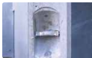
No concrete in the hole!
